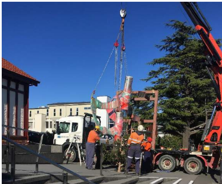
Accidental Intentions by James Mitchell Gifted by Robert G Hunt & Sally Mitchell Hunt MNZM Suter Patron, being installed by Scott Construction
